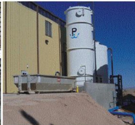
Vacuum Clarifier - Secondary Separation
