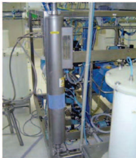
Figure 1. Installation of 7847 tube densitometer
